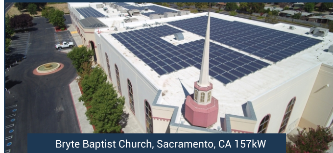
Church of the Foothills, Cameron Park, CA 127kW
